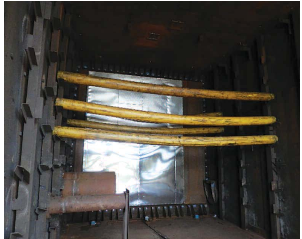
FireMaster vessel system installed on back wall of explosion chamber prior to explosion testing.
