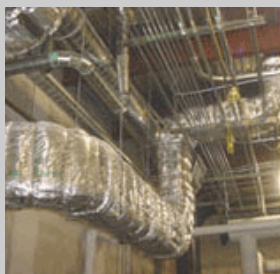
Grease ducts insulated with FireMaster Duct Wrap 2X2+ , allowing for zero clearance to combustibles and eliminating the need for gypsum chase constructions.
